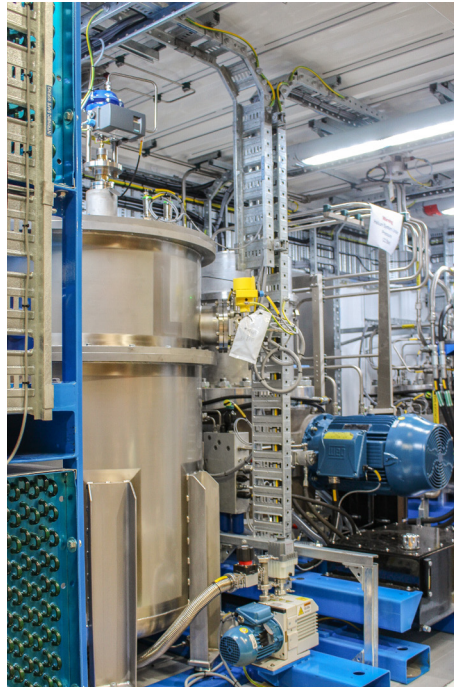
Hydrogen boil-off-gas management system
