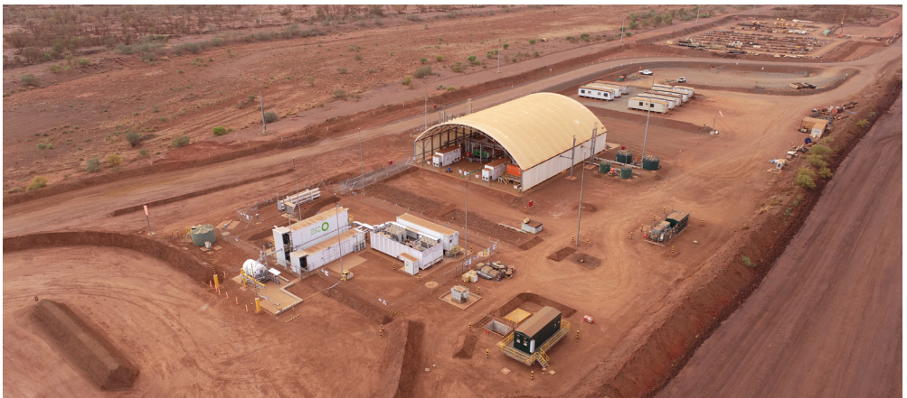
Hydrogen liquefaction plant at a mine site in Western Australia
